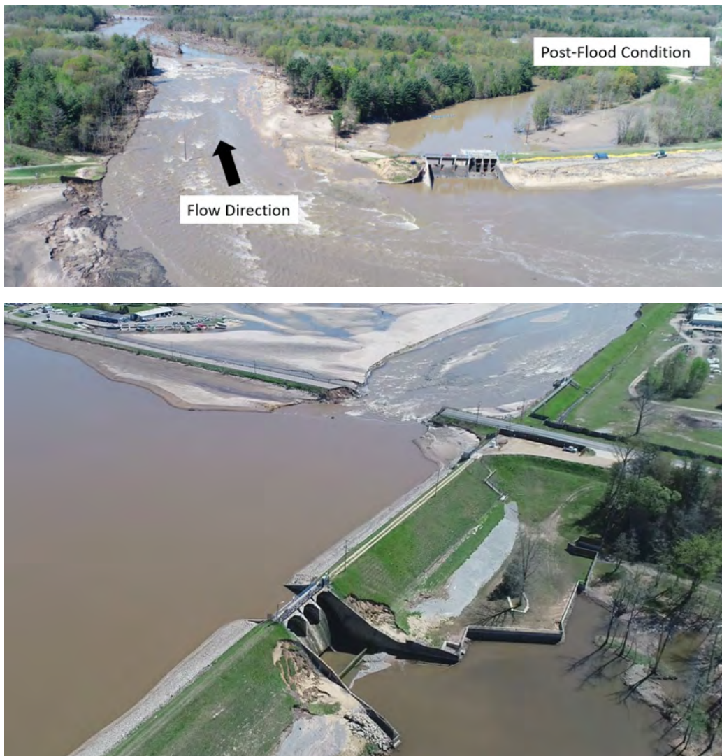
FIGURE 27: Aerial View of Edenville Dam Failure
