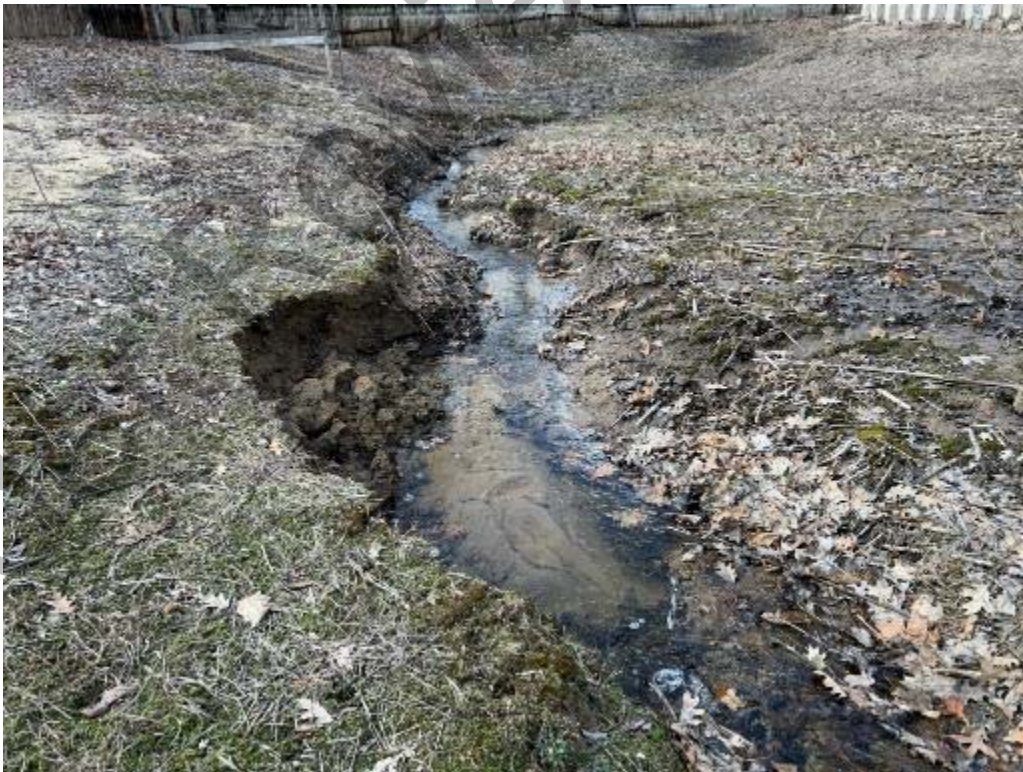
Site 16 – Bank erosion.
