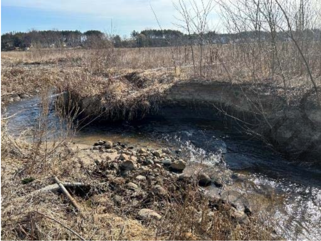
Site 1 – Looking downstream toward Tobacco River; headcutting and bank erosion.
