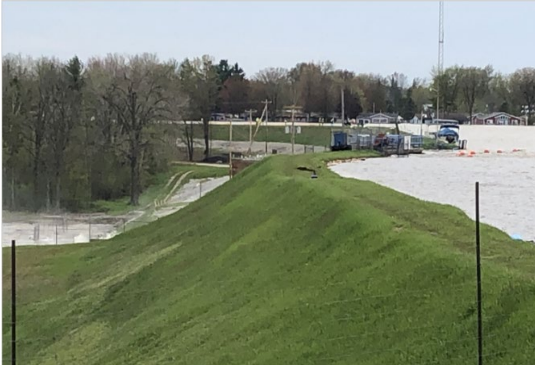
Figure 7: Photograph showing the downstream side of the Edenville left embankment at 5:31 p.m., Tuesday, May 19, 2020
