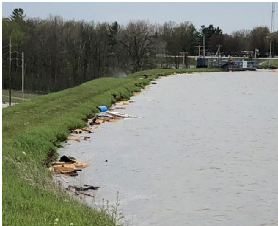
Figure 8: Enlarged photograph showing the upstream side of the Edenville left embankment at 5:31 p.m., Tuesday, May 19, 2020
