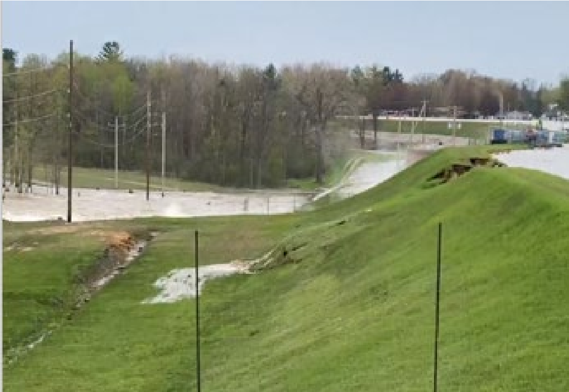
Figure 11: Enlarged still image from dam failure video at 6 seconds
