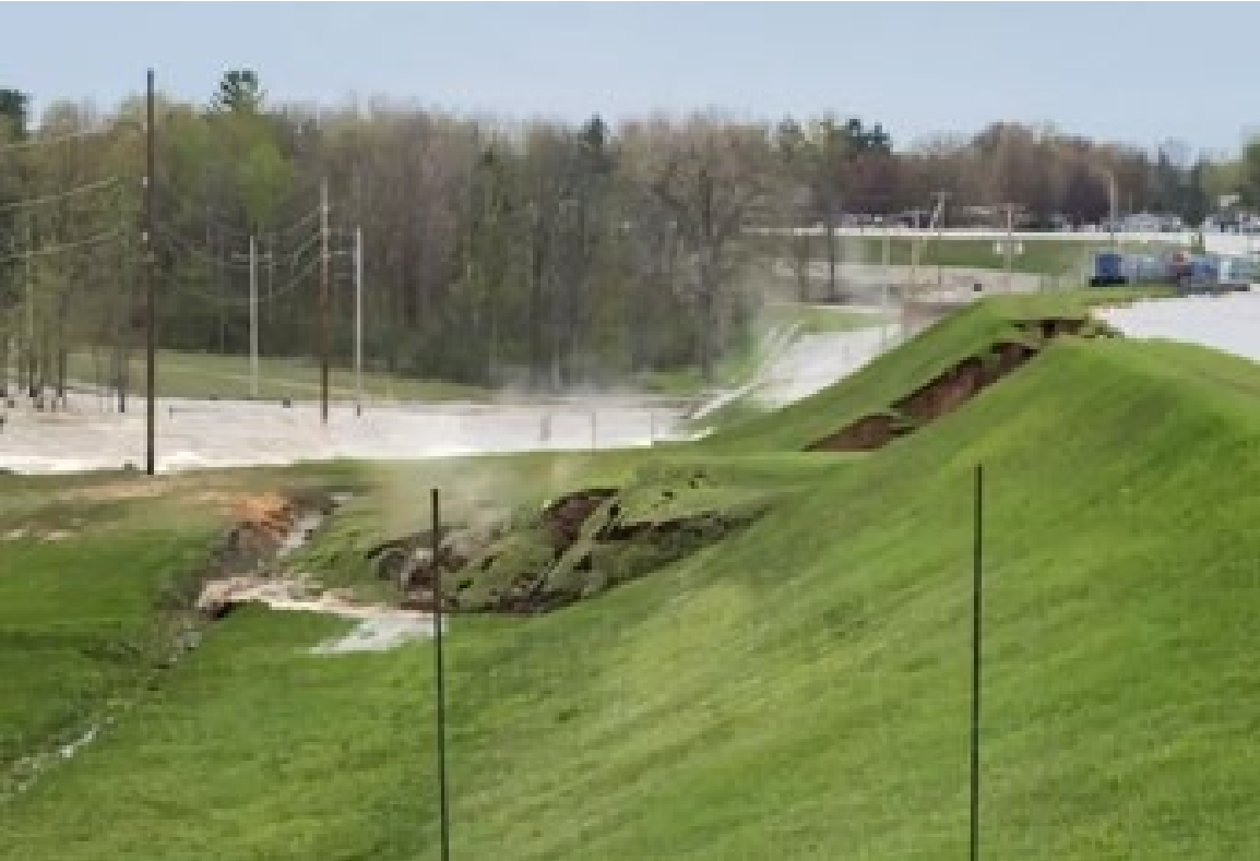
Figure 13: Enlarged still image from dam failure video at 8 seconds
