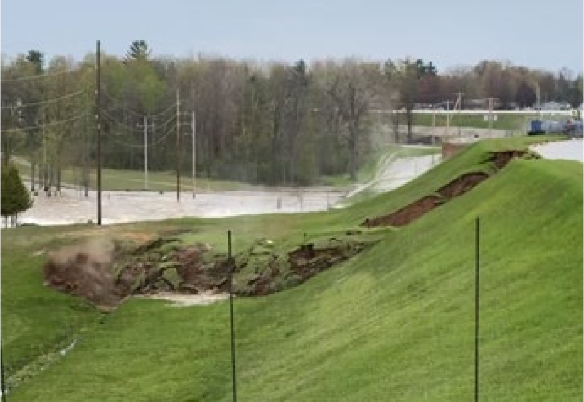
Figure 14: Enlarged still image from dam failure video at 10 seconds
