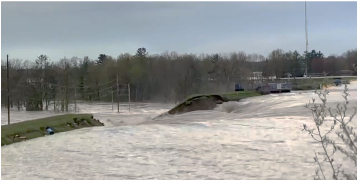
Figure 19: Edenville left embankment breach at 6:24 p.m. on Tuesday, May 19, 2020
