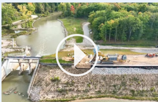
Click the image to watch a video of the Dewind One Pass trenching machine build the SCB wall.
