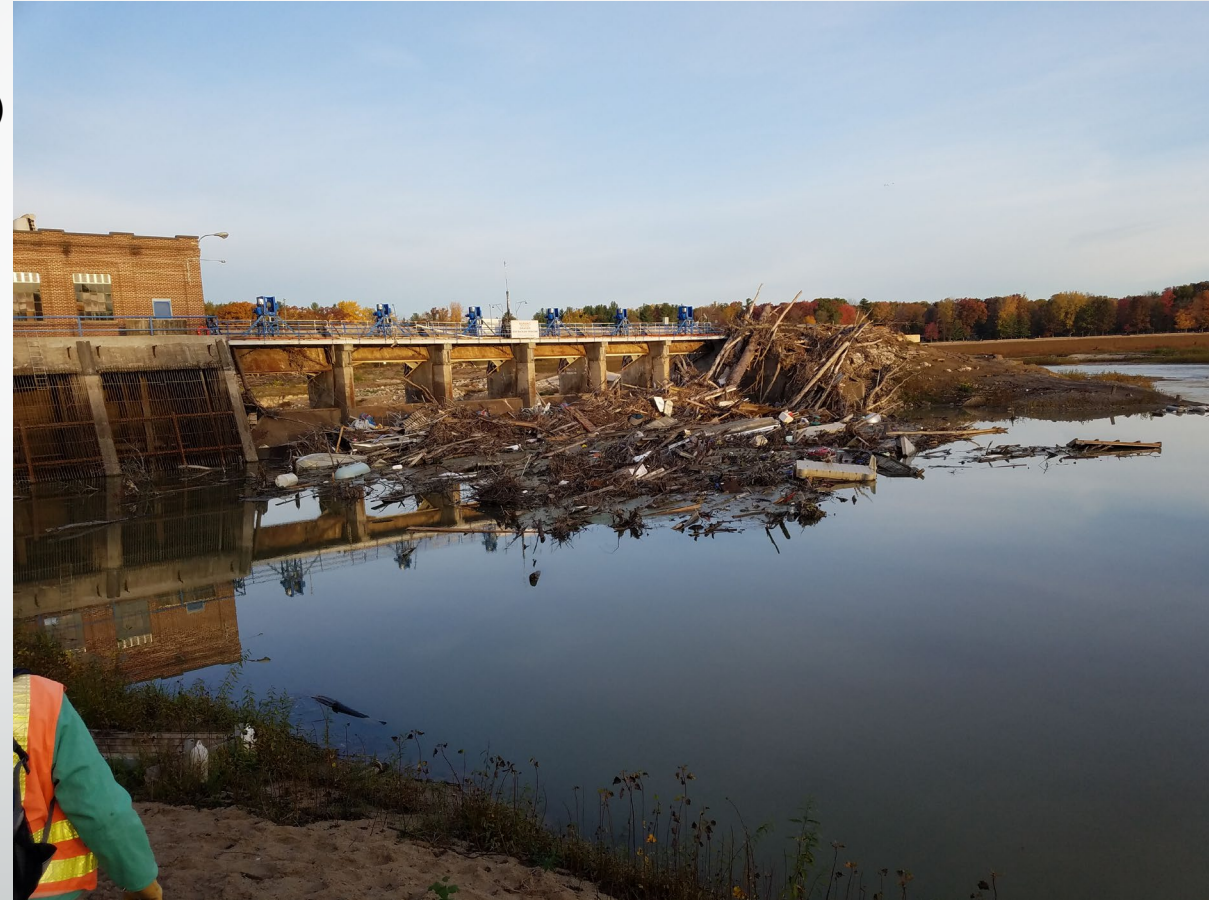
Sanford Dam – Debris accumulation on Dam, taken October 2020
