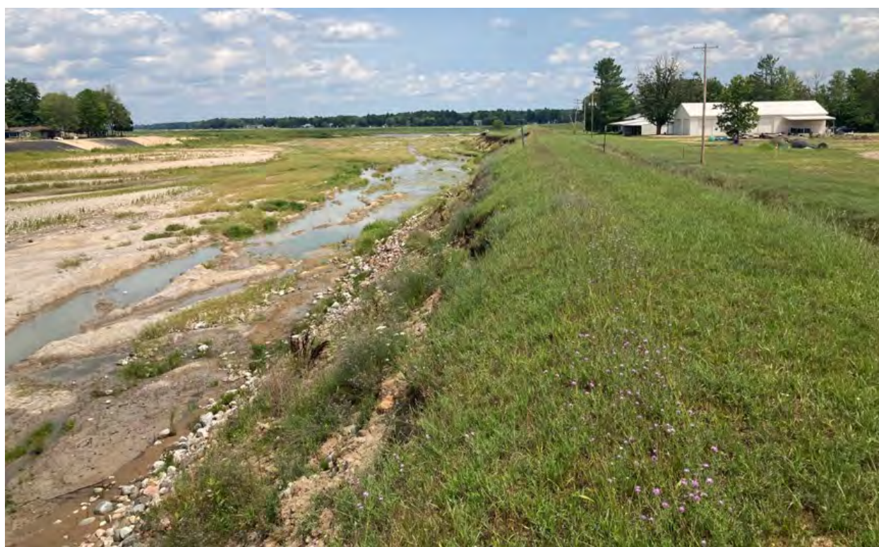
Photo 6. Right embankment overview facing east, on the east side of the Tobacco reach of the Edenville Dam.
