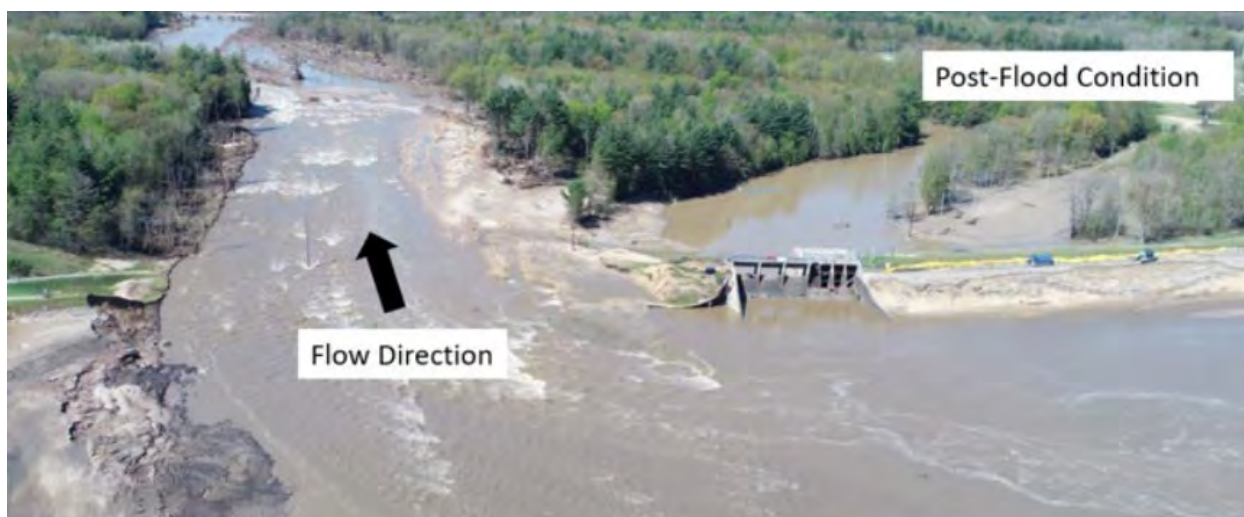
Photo 7. Edenville Dam Embankment Failure
