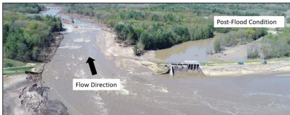
Exhibit 11 – Aerial View of Edenville Dam Failure
